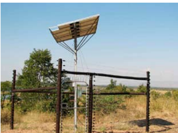
A newly installed Solar power supply.
